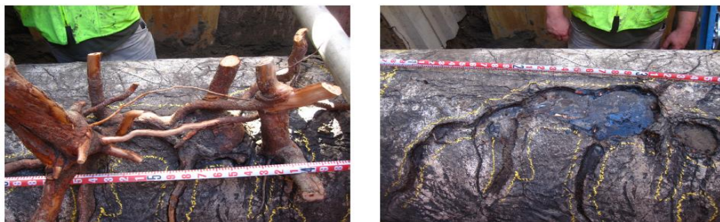
Examples of tree roots interacting with the natural gas transmission pipeline and causing damage to the protective coating.
